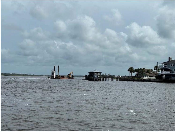
Photo 5: 20' Wide Push Barge motoring to Baseline 7, where the barge was actively dredging.
