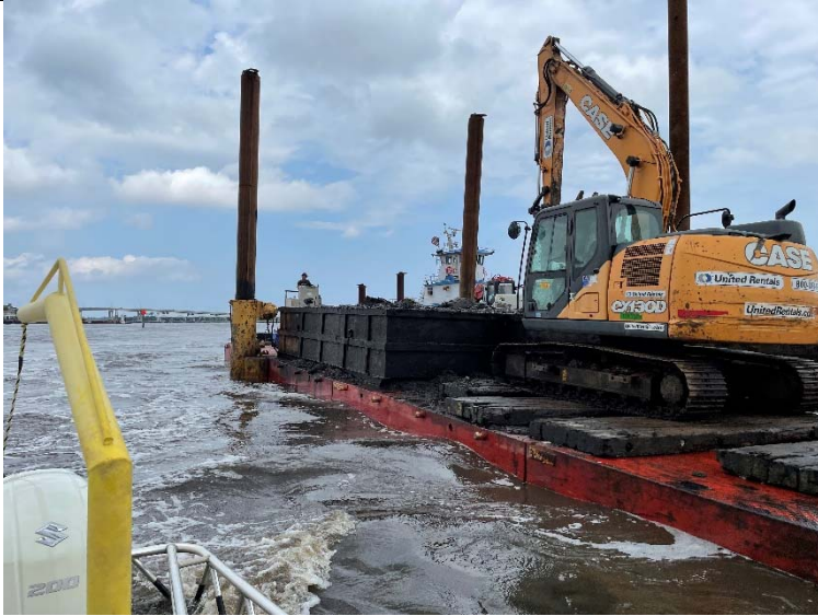
Photo 3: Additional photo of 26' Thruster Barge full of material off-loading to the Hopper storage barge.
