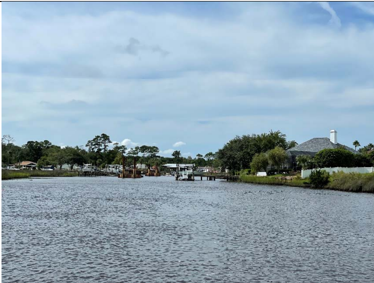
Photo 1: View of two 20' Wide Push Barge located in Baseline 1: Southern IOP
